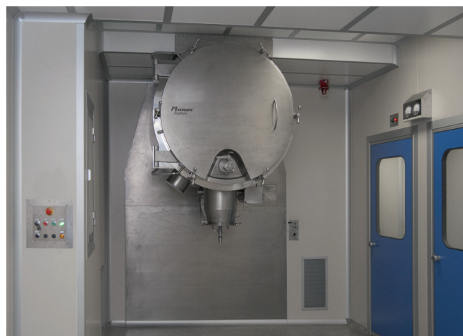
Installation in clean room
