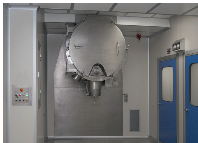
Installation in clean room
